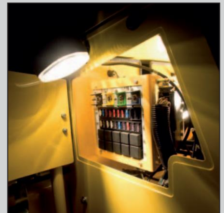
The fuse box – well protected yet readily accessible.
