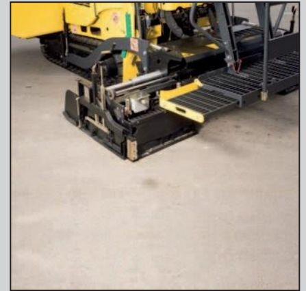
Together with the screed, the operator's platform can also be adjusted to site conditions with laterally shifting consoles.
